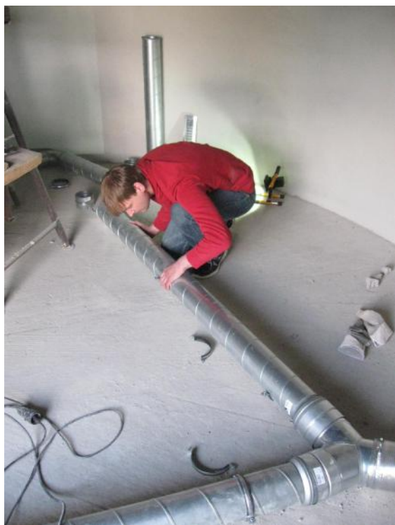
Figure 16: Installation of the ventilation pipes in the telescope room. The system will be installed under a wooden ceiling.
